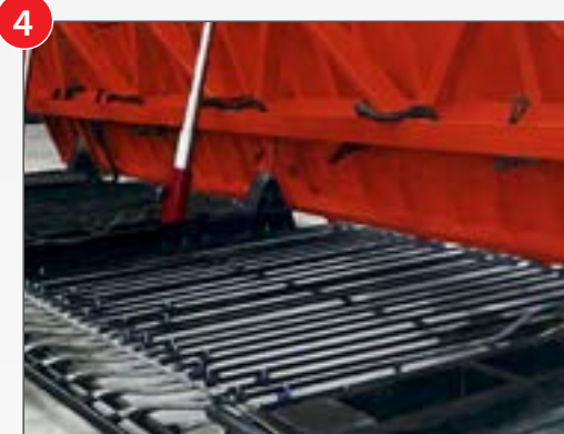
4 A hot water, closed-loop piping system provides the radiant heat element under the form.
