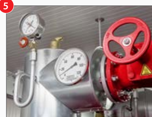
5 The system achieves a maximum concrete temperature of 50 °C to 70 °C with water temperatures of 80 °C to 110 °C.
